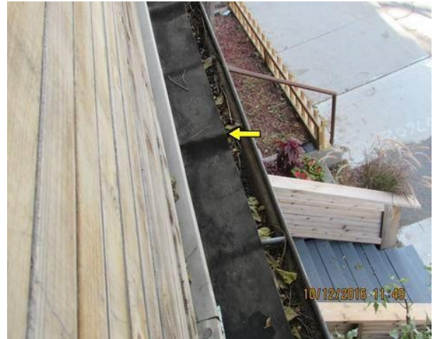
Buckled membrane under second floor decking at front of house
