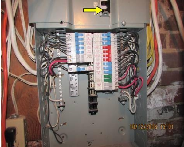
Electrical panel and main shut off
