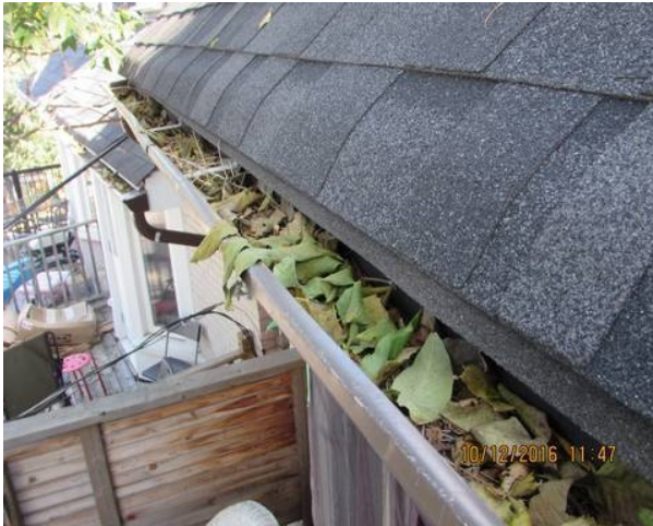
Gutters full of debris
