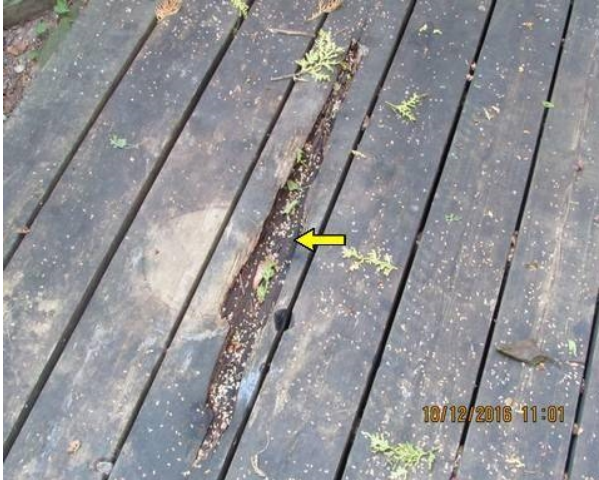
Rotted deck boards
