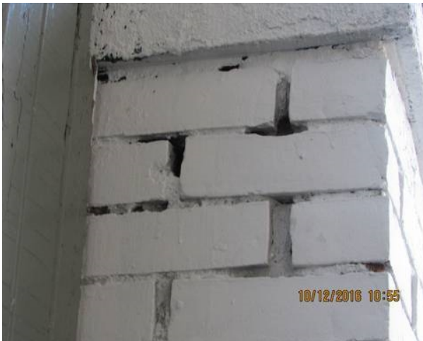
Mortar deterioration at column
