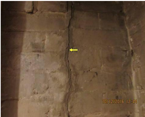
Crack in wall
