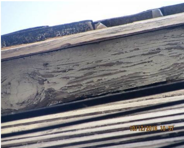
Peeling paint on soffit
