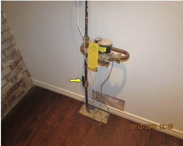
Water meter and main shut off
