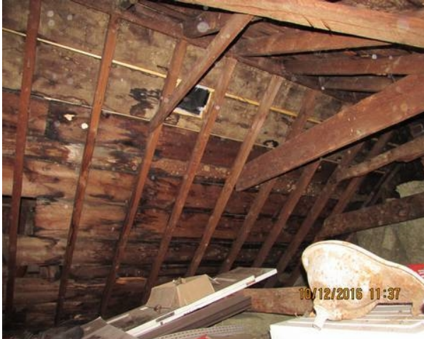
Staining on sheathing
