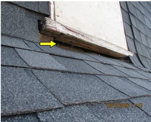
Opening under boarded up attic window
