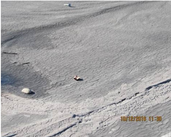
Deteriorated flat roof membrane
