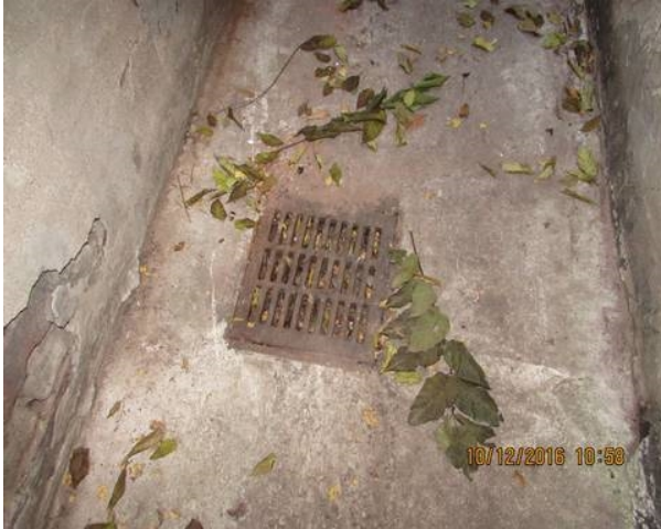
Drain clogged with debris
