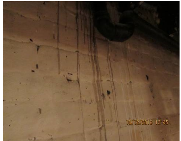
Staining on wall
