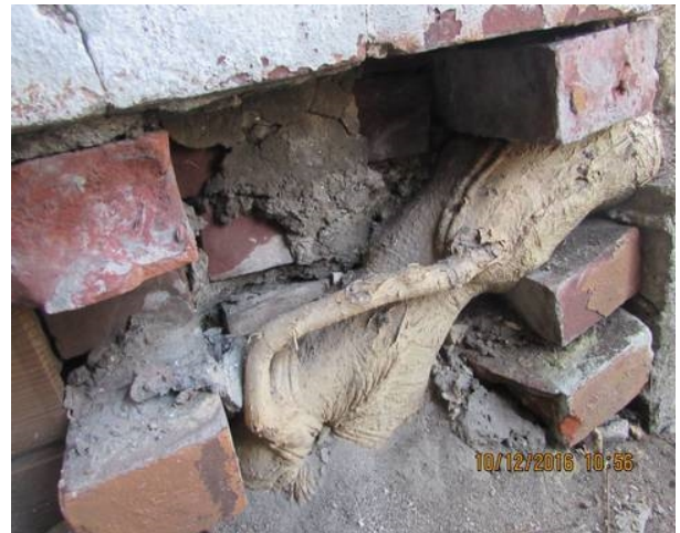
Tree growing out of base of damaged column
