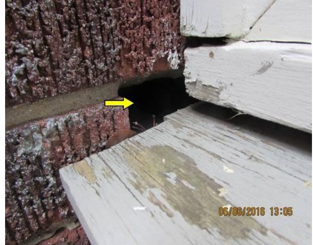
hole in exterior wall
