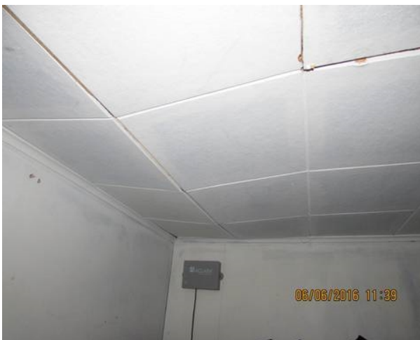
Sagging in ceiling tiles
