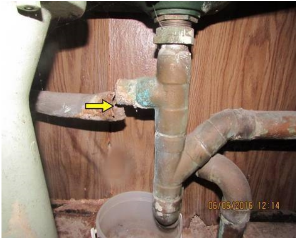
Corroded and disconnected pipe
