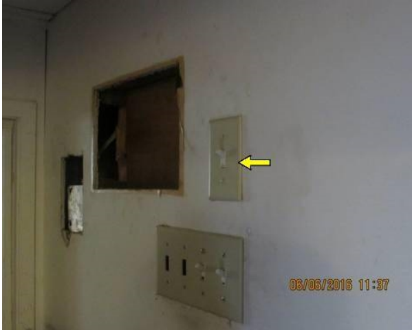
Furnace shut off
