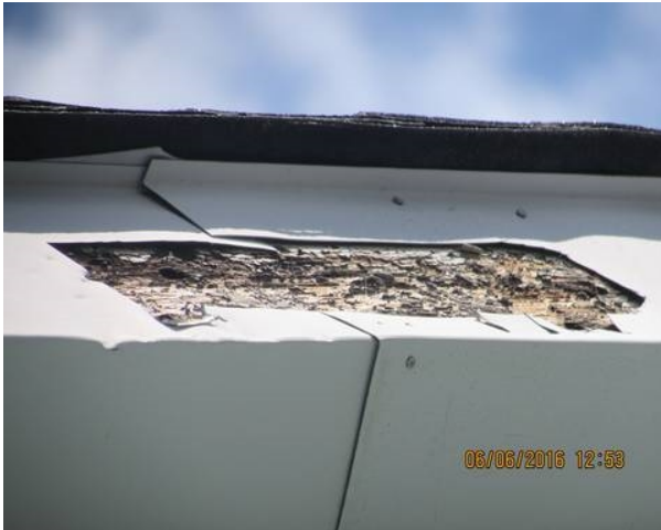
Wood fascia exposed
