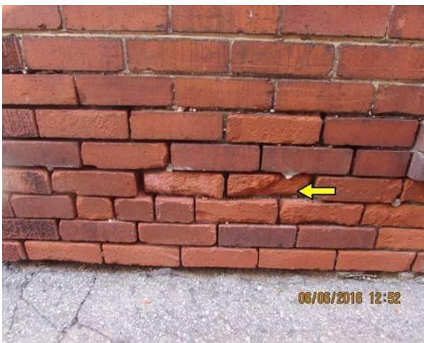
Deteriorating brick and mortar
