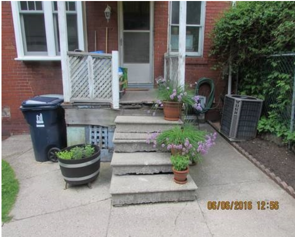
Missing hand rail
