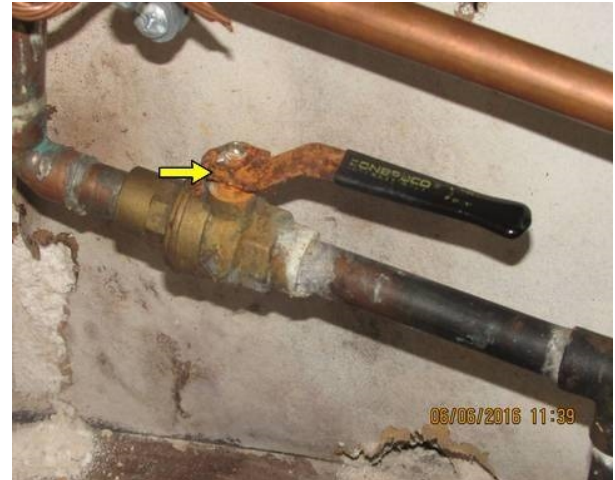
Corroded shut off handle
