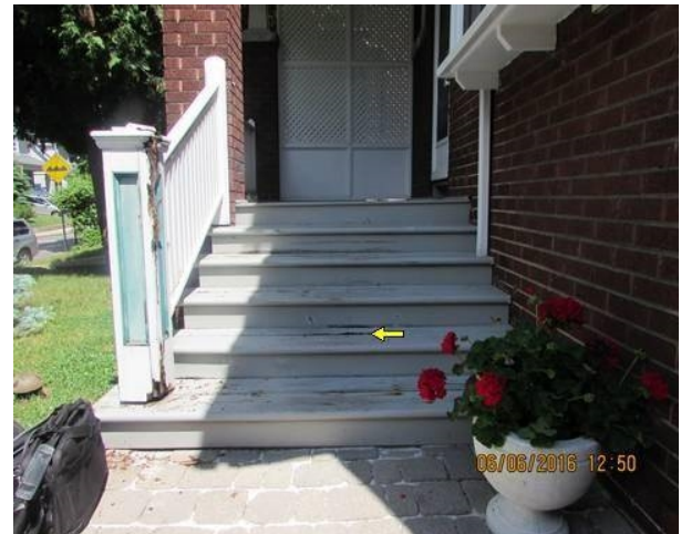
Boards are rotting
