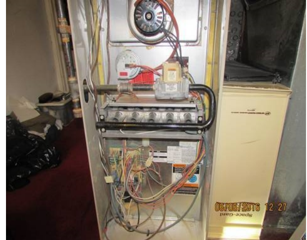
Mid efficiency furnace
