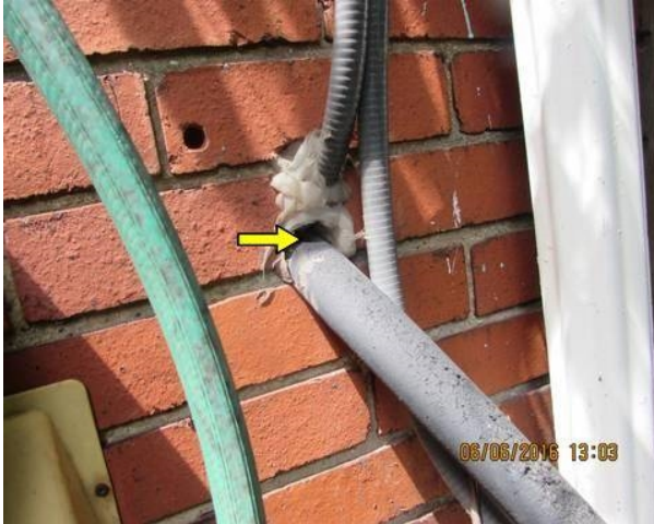
Hole in exterior wall
