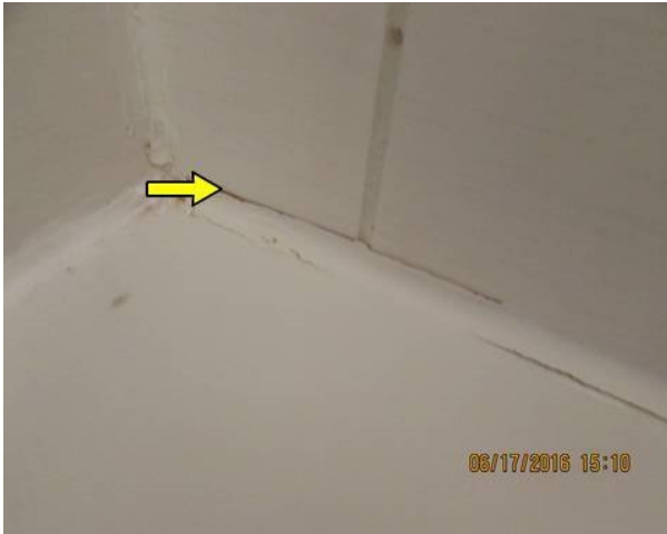
Deteriorating caulking at tub surround
