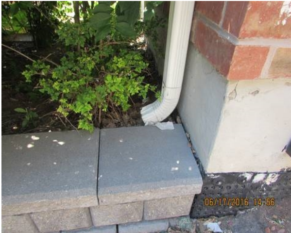
Downspout discharging against foundation
