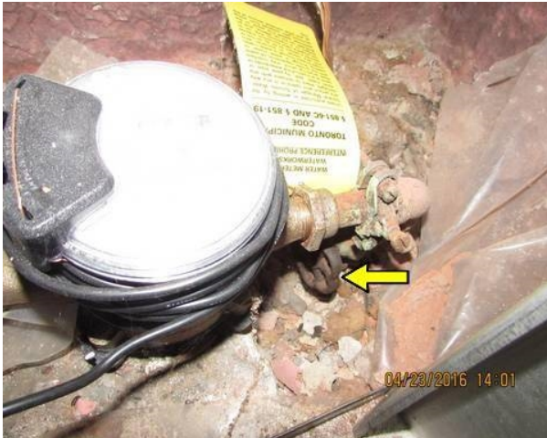
Water meter and main shutoff
