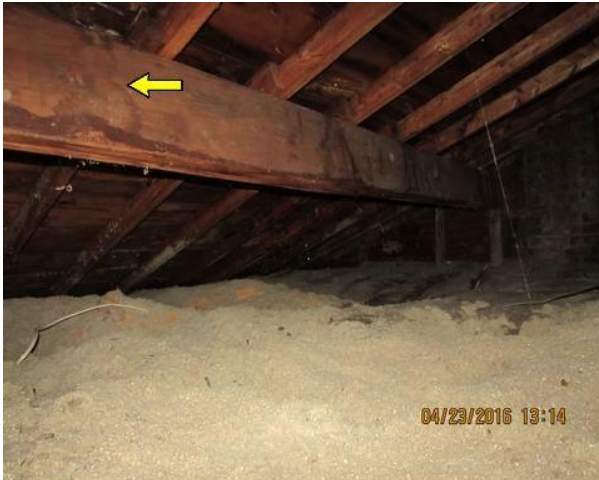
Water staining on beam
