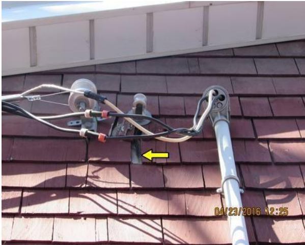
Missing wood siding
