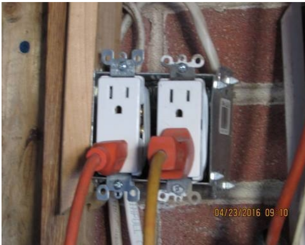
Missing receptacle cover
