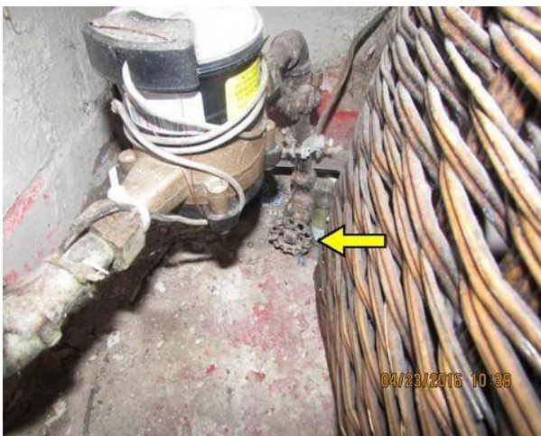
Water meter and main shutoff
