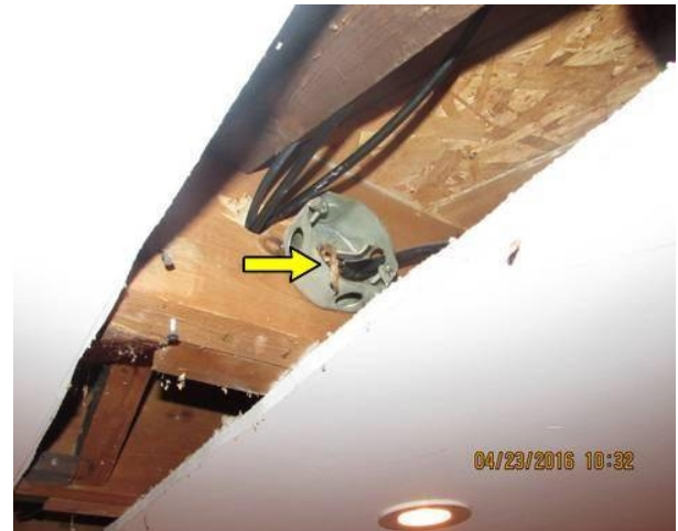
Exposed wires and missing junction box cover
