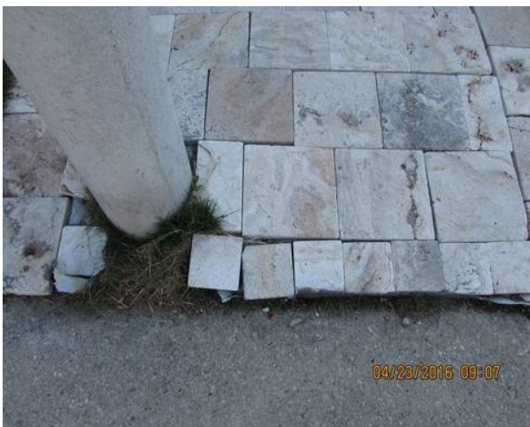
Loose and uneven walkway tiles
