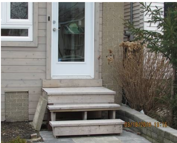
Add handrail for safety
