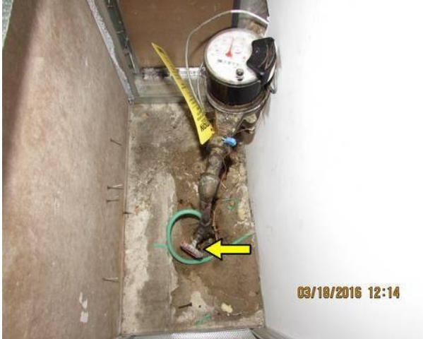
Water meter and main shut off
