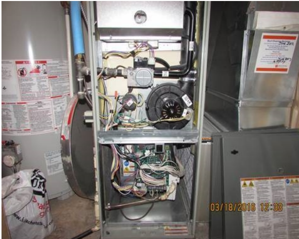
High efficiency furnace
