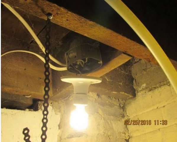
Light fixture not secured
