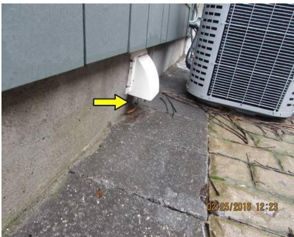
Dryer vent to close to grade
