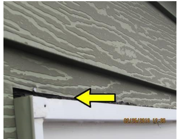
Gap between window and siding where water can penetrate
