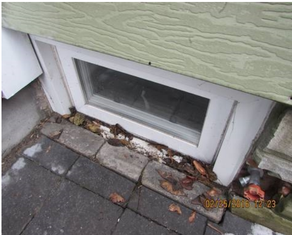
Window too close to grade
