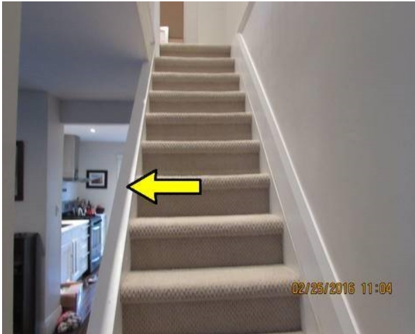
Missing guard and handrail
