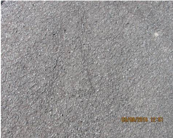
Upper Flat roof membrane cracking
