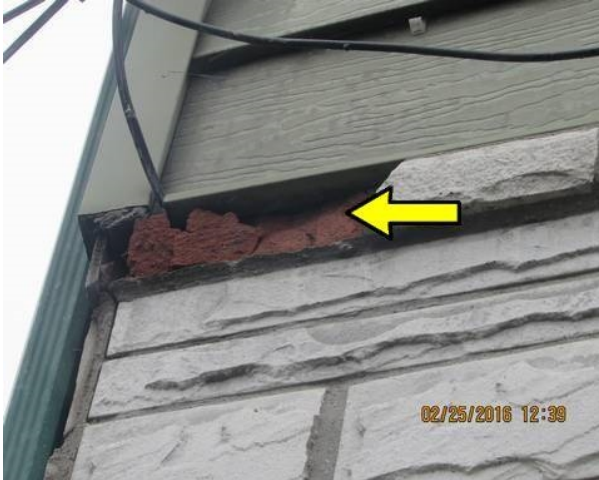
Damaged brick siding
