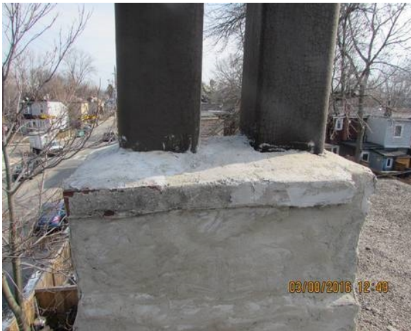
Chimney cap recently parged
