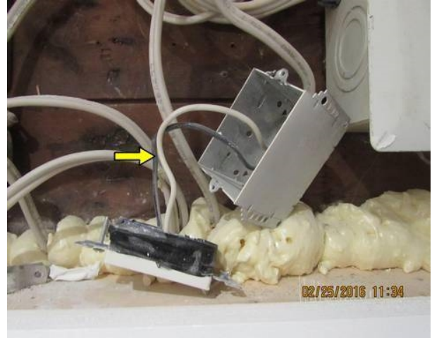
Exposed receptacle wires
