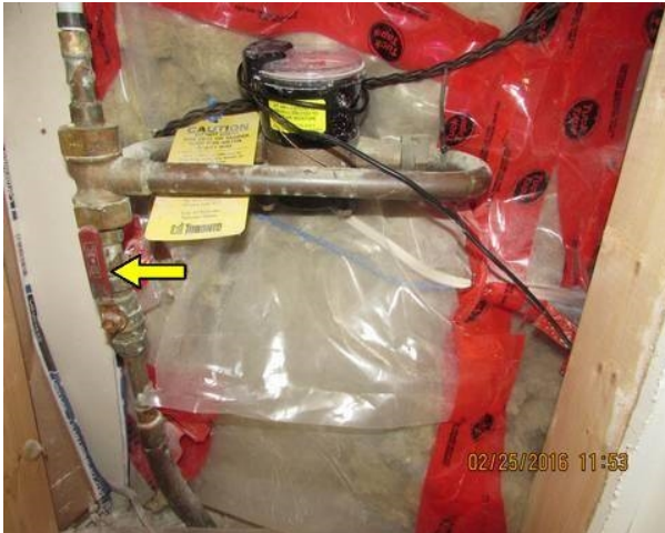
Water meter and main shut off
