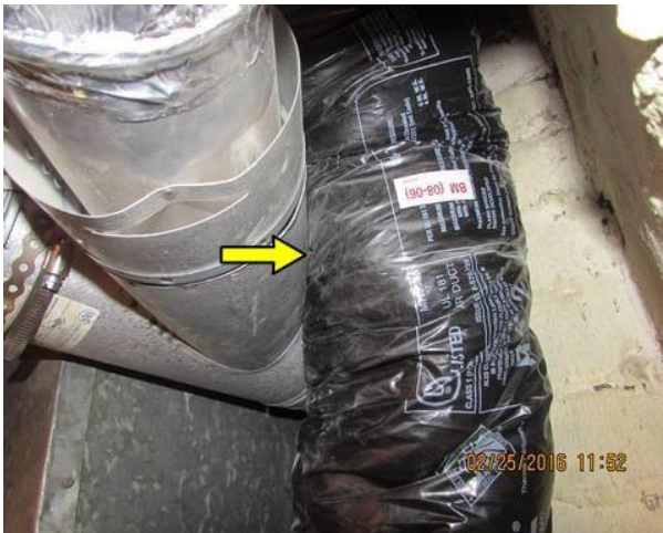
Plastic pipe wrap resting on heating vent. Provide separation here.
