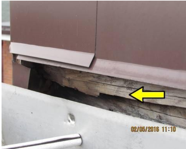
Rotted fascia board
