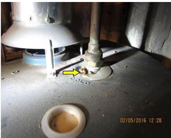
Burnt plastic at top of water heater
