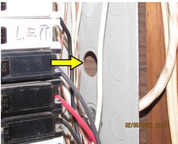
Missing grommet in electrical panel
