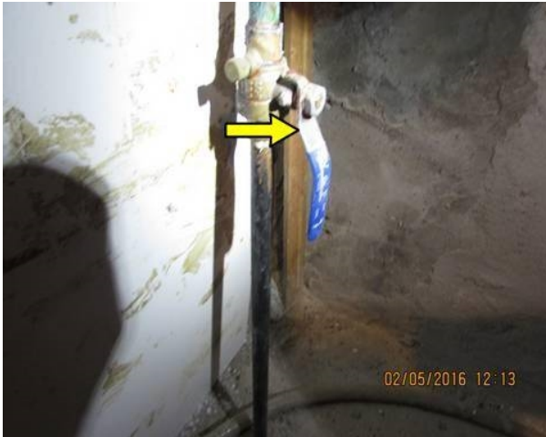
Water main shut off
