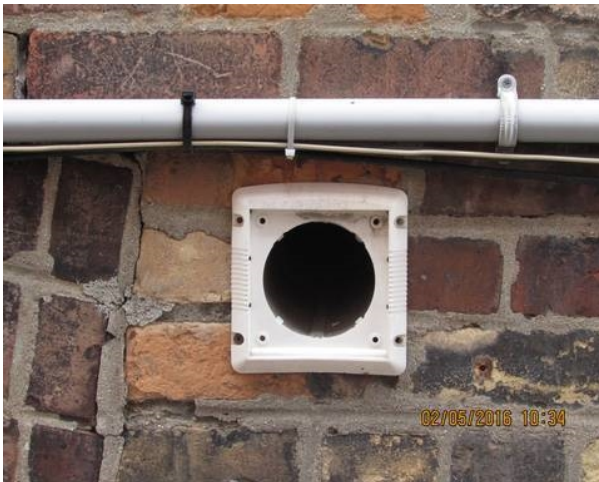
Missing vent cover
