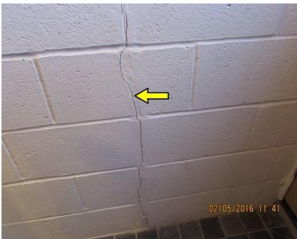
Settlement crack at basement walkout
