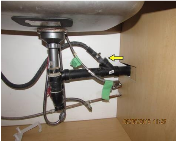
Dishwasher drain on wrong side of trap
