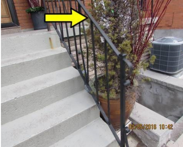
Handrail is loose
