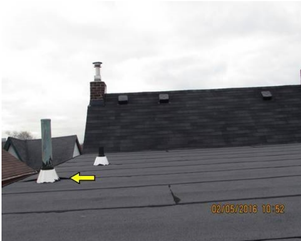
Roofing material is not caulked
