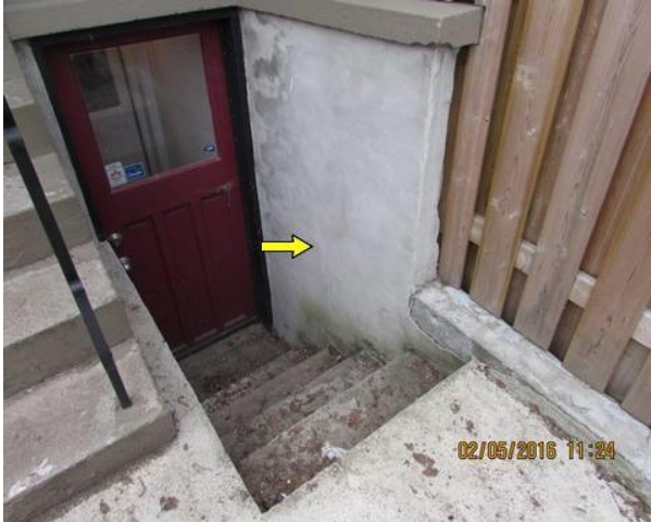
Add handrail here
