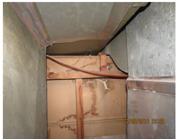
Water stains on drywall behind furnace
