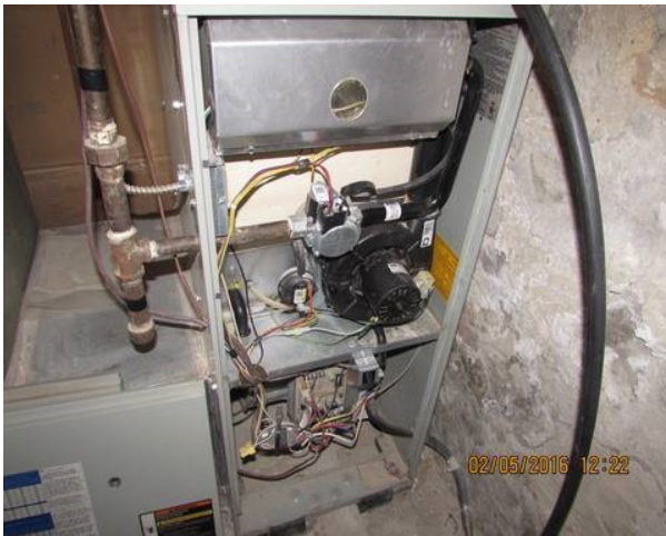
High efficiency furnace
