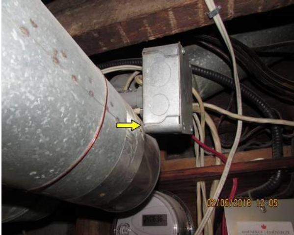
Electrical junction box resting on duct
