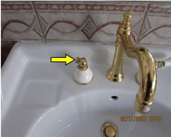
Missing handle for hot water
