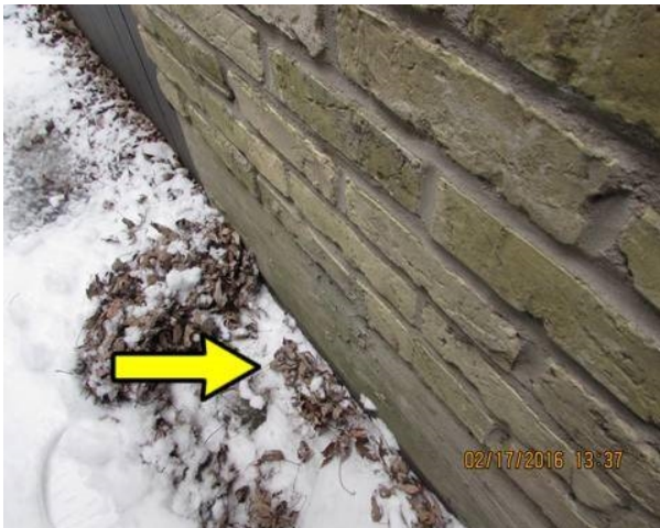
Grade slopes toward building here. North east corner
