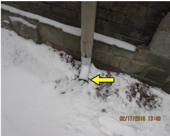
Downspout discharging to close to the foundation
