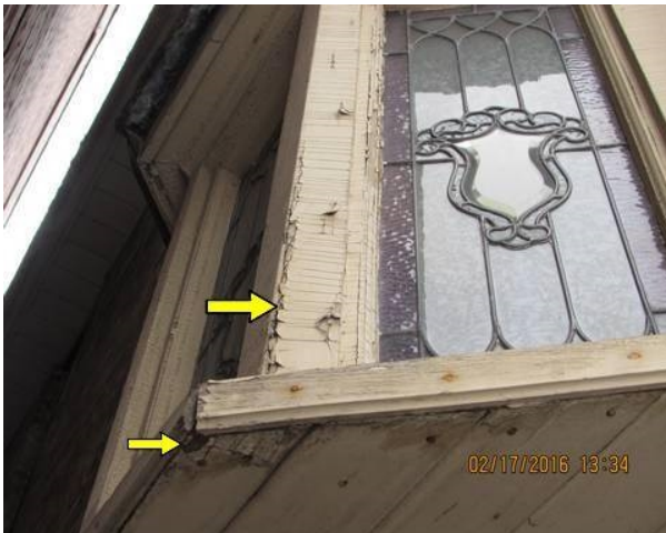
Deteriorating paint around window
