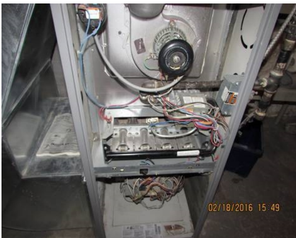
Mid efficiency furnace
