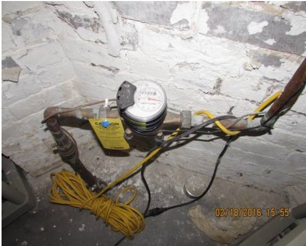
Copper water main, Main shut off and meter
