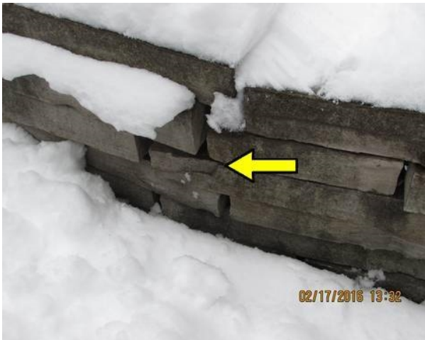
Retaining wall movement
