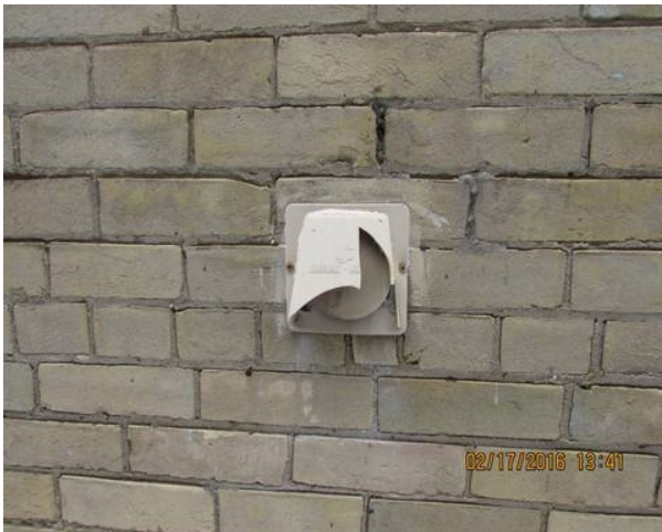
Broken dryer vent cover
