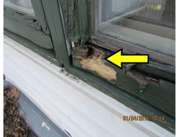
Rotted window frame
