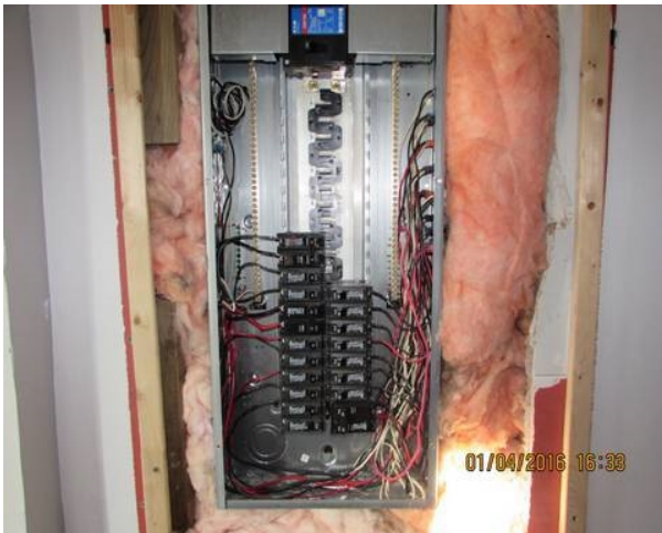
200 Amp electrical panel
