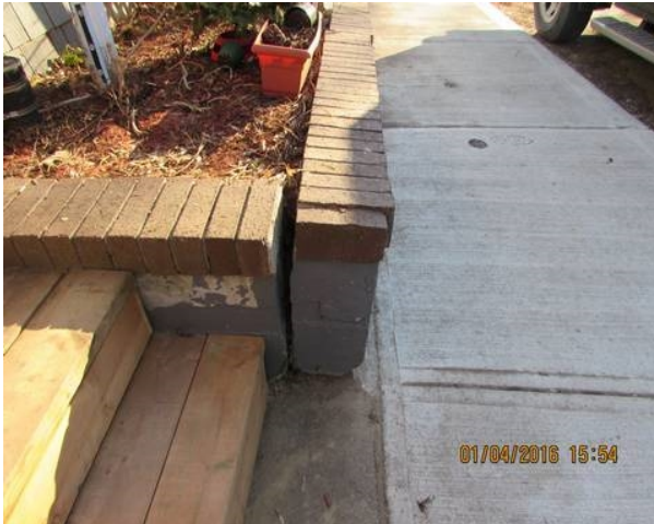
Retaining wall leaning slightly
