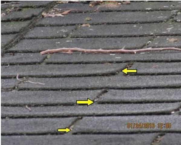
Shingles starting to show signs of wear.
