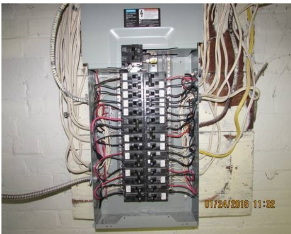
Electrical panel. 100 Amp service
