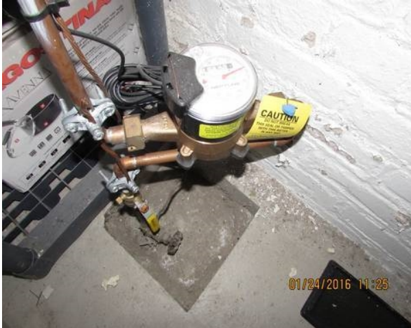
Water meter and main shut off. Lead supply.
