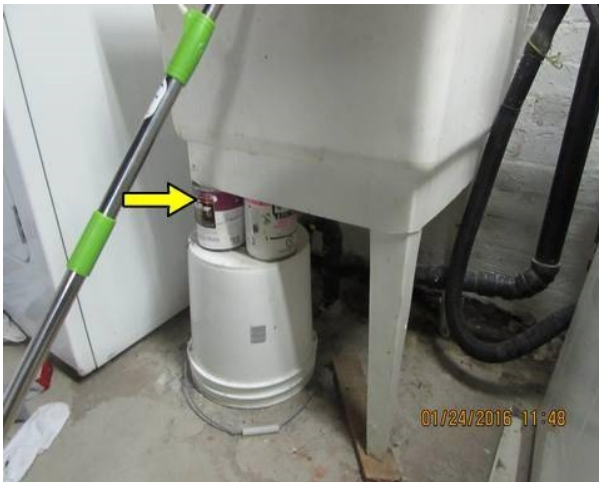
Damaged laundry tub. Leg missing.
