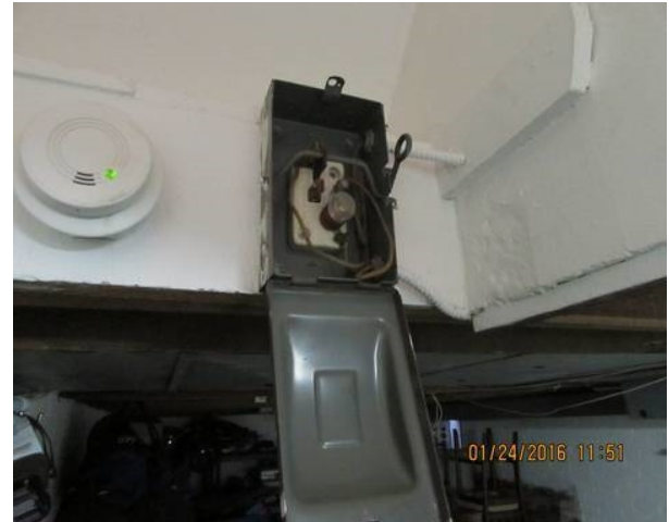
Obsolete glass fuse breaker panel used for furnace.
