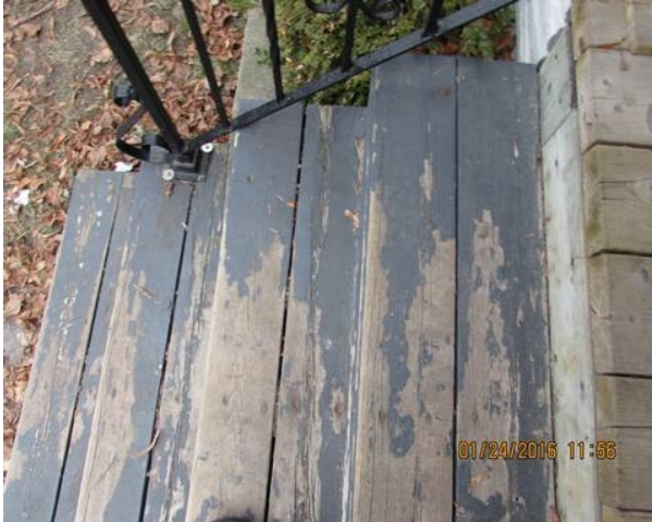
Peeling paint at porch steps
