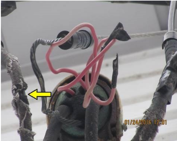
Deteriorated sheathing on entrance cable.
