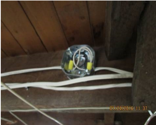
Missing cover on junction box
