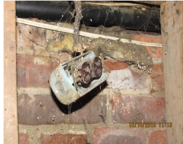
Electrical outlet hanging from the ceiling
