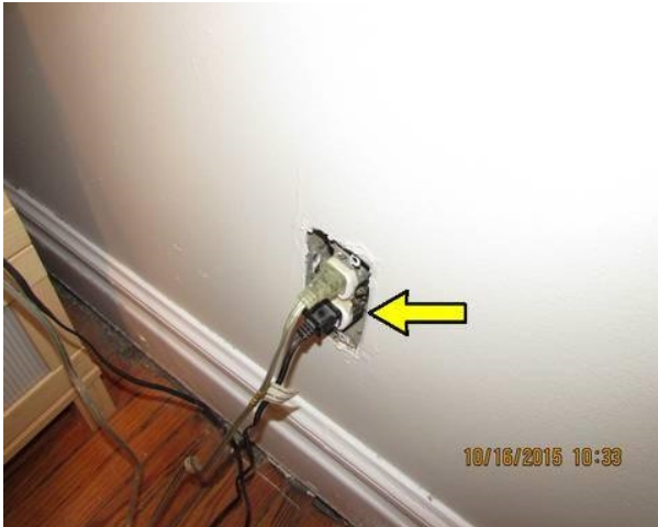
Missing cover plates
