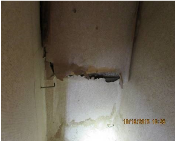
Damage found inside bedroom closet
