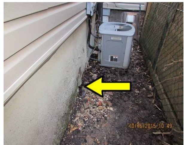
Improve grading and repara foundation in this area
