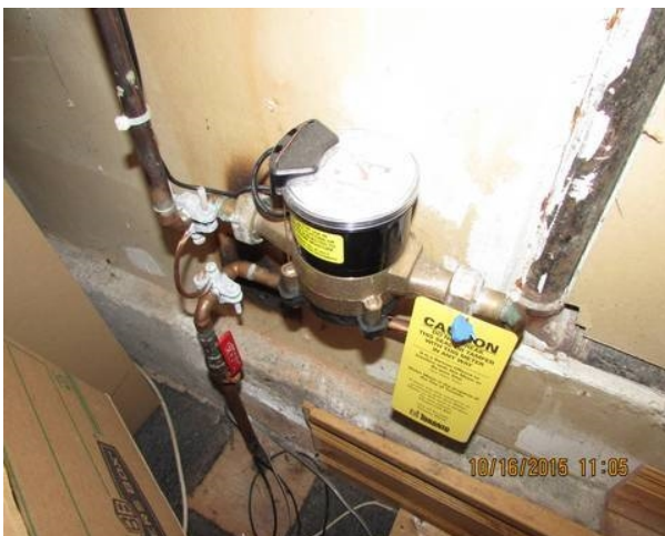
Water meter and main shut off
