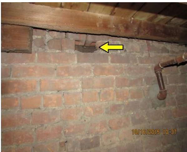
missing brick under porch
