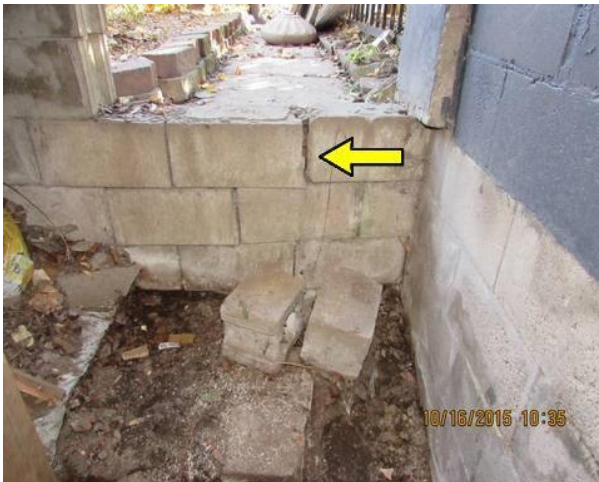
Wall is leaning slightly.
