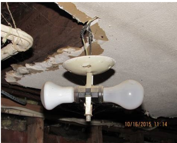
Light fixture not secured
