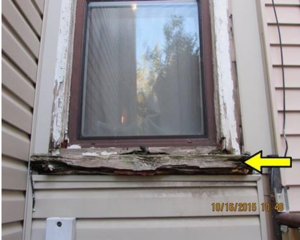
Rotted window frames
