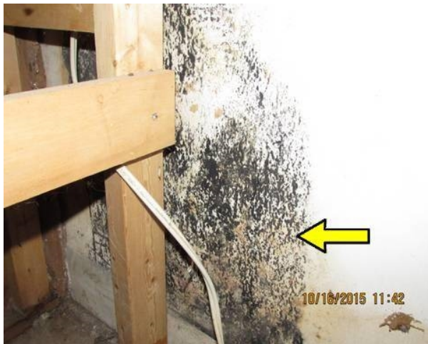
Staining on basement wall
