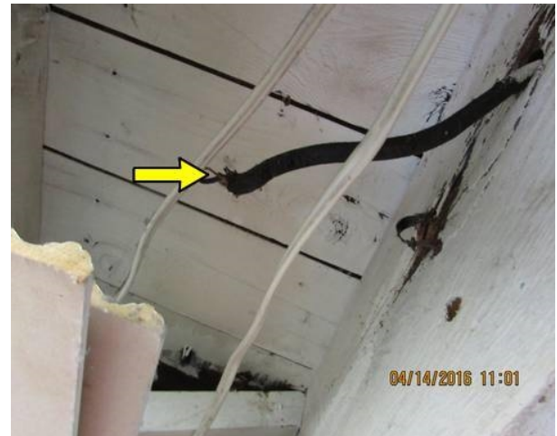
Unterminated and exposed electrical wire
