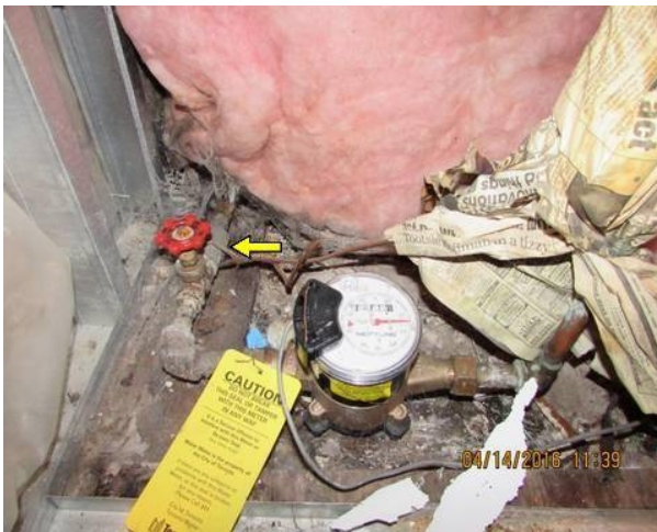
Missing ground clamp
