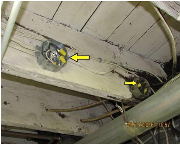
Missing covers on junction boxes
