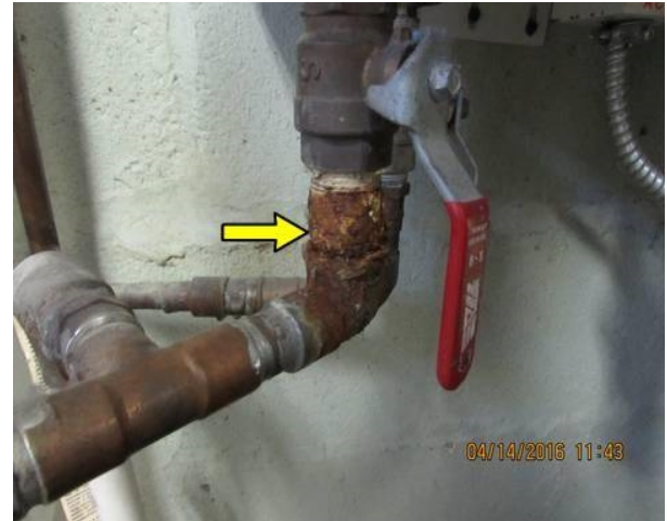
Corrosion on water line
