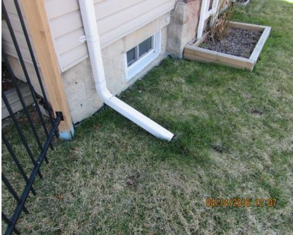
Downspout discharging to close to foundation
