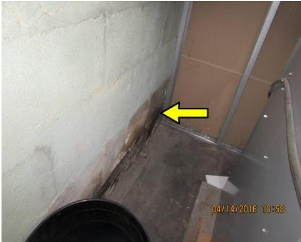
Staining on wall behind furnace
