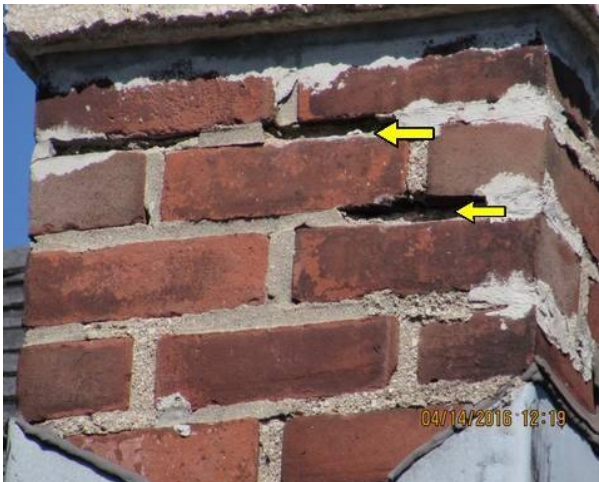
Mortar deterioration at abandoned south chimney
