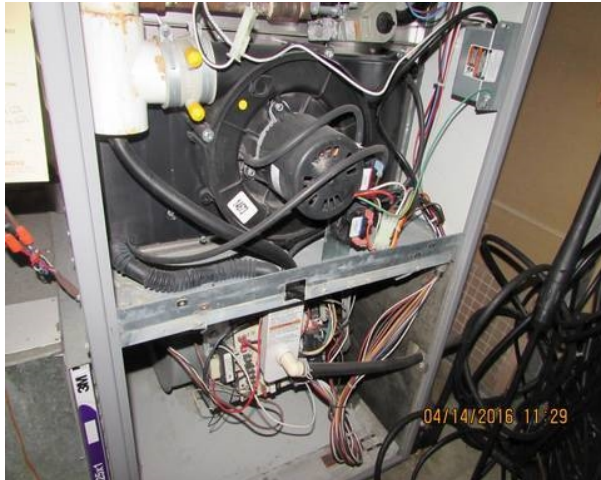
High efficiency furnace
