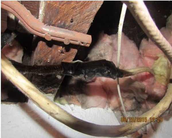
Spliced connections should be inside a junction box.
