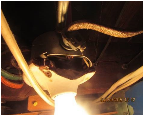
Broken light cover and exposed wires
