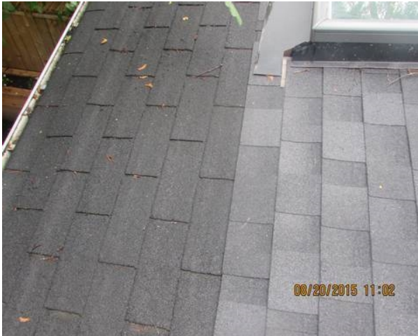
Deteriorating shingles over kitchen
