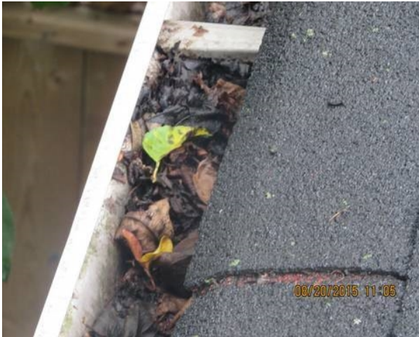
Gutters filled with debris
