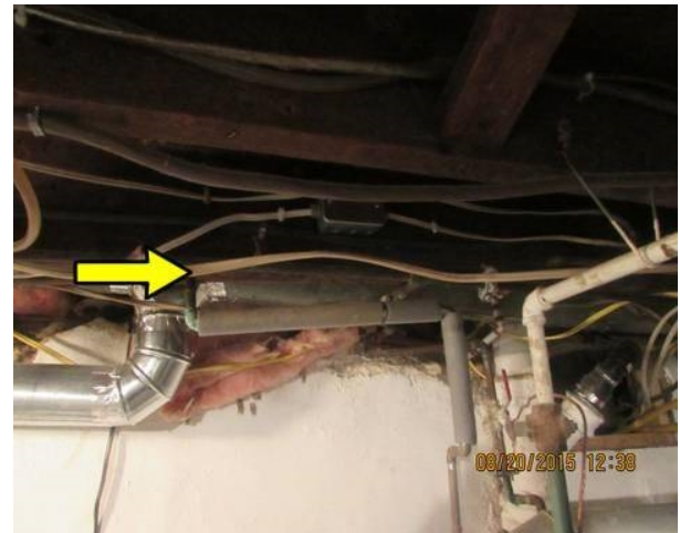
Secure loose wires
