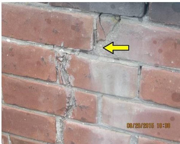
Settlement crack under front window
